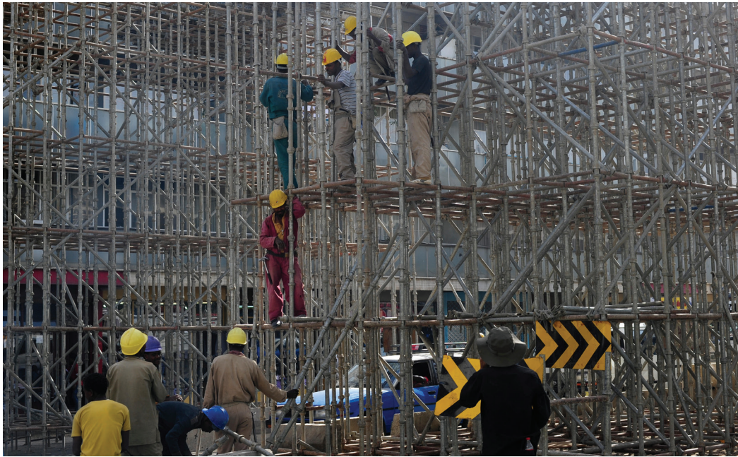
THE BUILDING OF INFRASTRUCTURE IN AFRICA, LIKE THIS LIGHT RAIL NETWORK BEING BUILT IN ADDIS ABABA BY A CHINESE COMPANY, IS ESSENTIAL FOR PROMOTING TRADE AND DEVELOPMENT.
